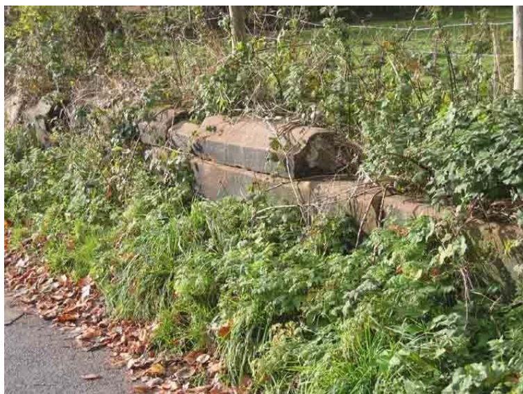
Damage to wall around Lunt Green on Lunt Lane
